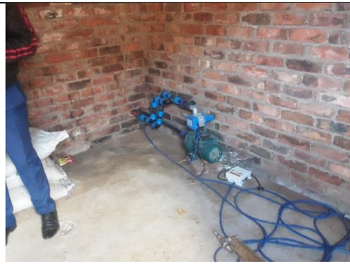
Fig.4.16: Storage Building with borehole pump
