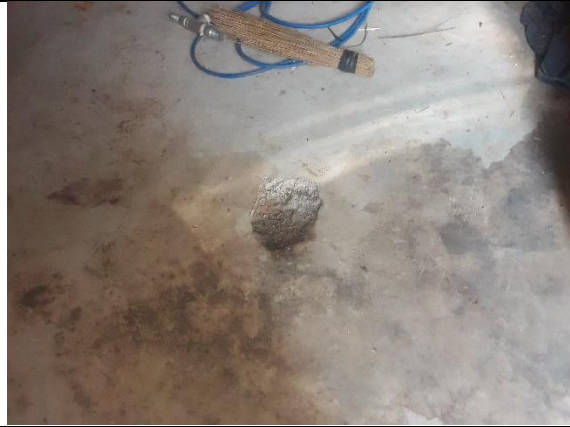
Fig.4.14: Storage Building floor minor damages to be fixed
