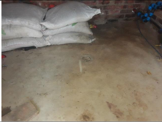
Fig.4.13: Storage Building floor minor damages to be fixed
